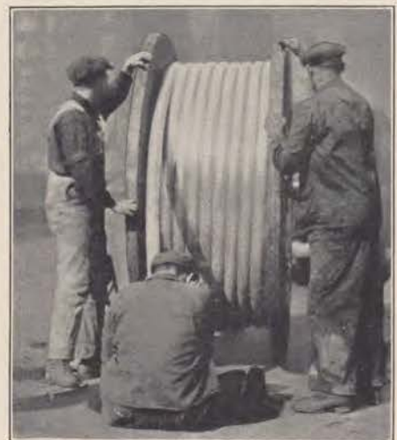
In this familiar scene the telephone wires are being put underground, enclosed in their protective sheath of lead.
