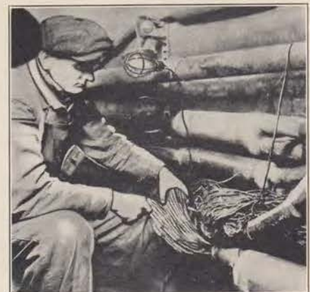
Solder joins the wires in lead covered cables and also joins the lead sheaths where two cables come together, thus preventing moisture from creeping in to injure the insulation.
