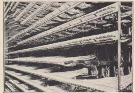
Thousands of pounds of purified cotton and silk insulation, frequently impregnated with cellulose acetate lacquer, are used on the wires and cables in the telephone exchange to connect together the switchboards and auxiliary apparatus.
