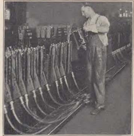
Asphalt in cable terminals, used when telephone wires are joined to a lead covered cable, prevents moisture working in among the wires.
