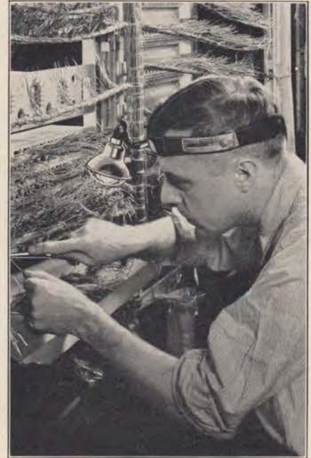
This installer is connecting up the cotton and silk covered copper conductors in the telephone switchboard.
