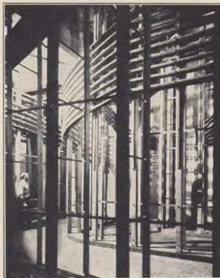
A cable vault located far below a city street. Here is an orderly array of myriad telephone wires collected into cables and sheathed in coats of lead and antimony.
